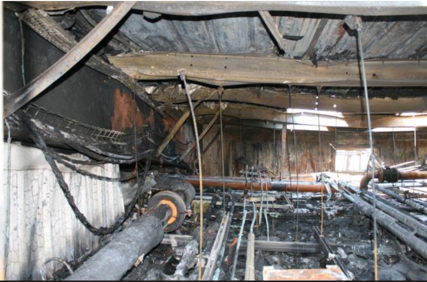
Roof void damage after fire
